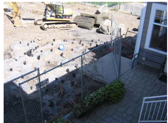
Blastholes were located within 7-ft of the plate glass door of the Dentist's office (above, right side of photograph).
